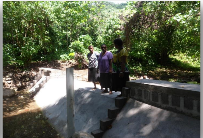
New Damp for Mapbest Coop Hydro Project with compliment of our VSA, Steffen Gnatzy.
